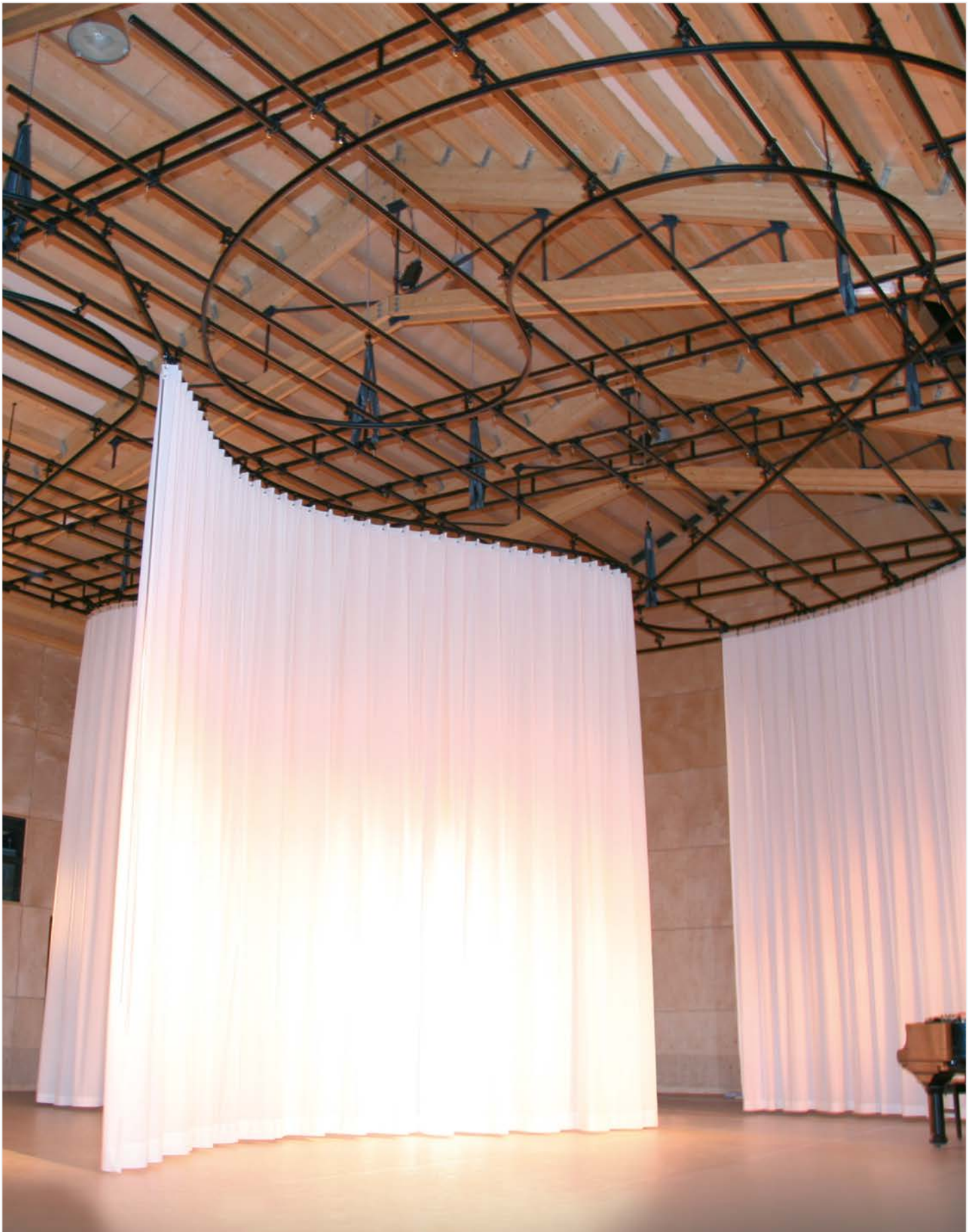
//Photo: O.T. Theater – Rotterdam, Netherlands / TRUMPF 95 curtain track, complex configuration maximizes the versatility of the avant-garde, ultra-simple performance space
