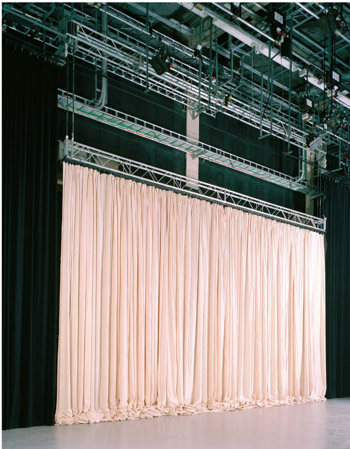
//Photo: WDR TV-Studio – Cologne, Germany / TRUMPF 95 tracks with motorized truss/track dropout section
